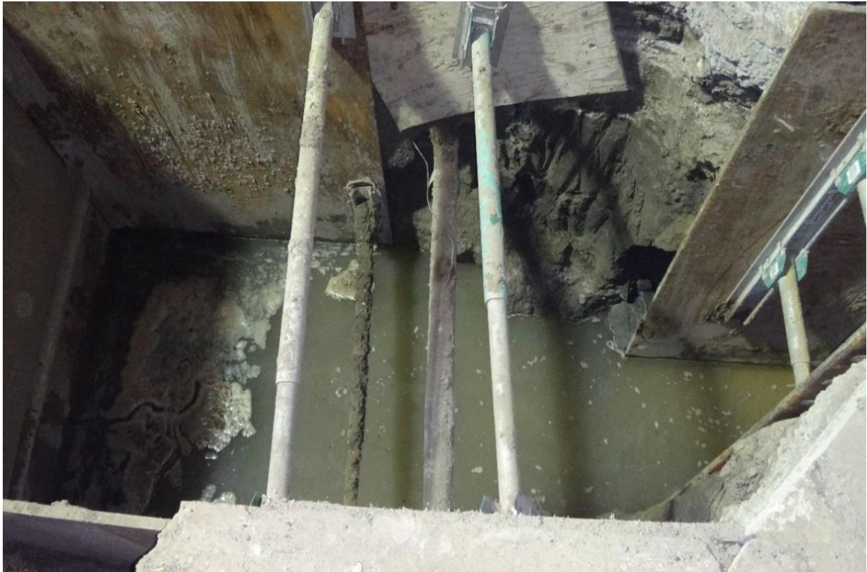
Figure 9: Groundwater Encountered During Excavation
