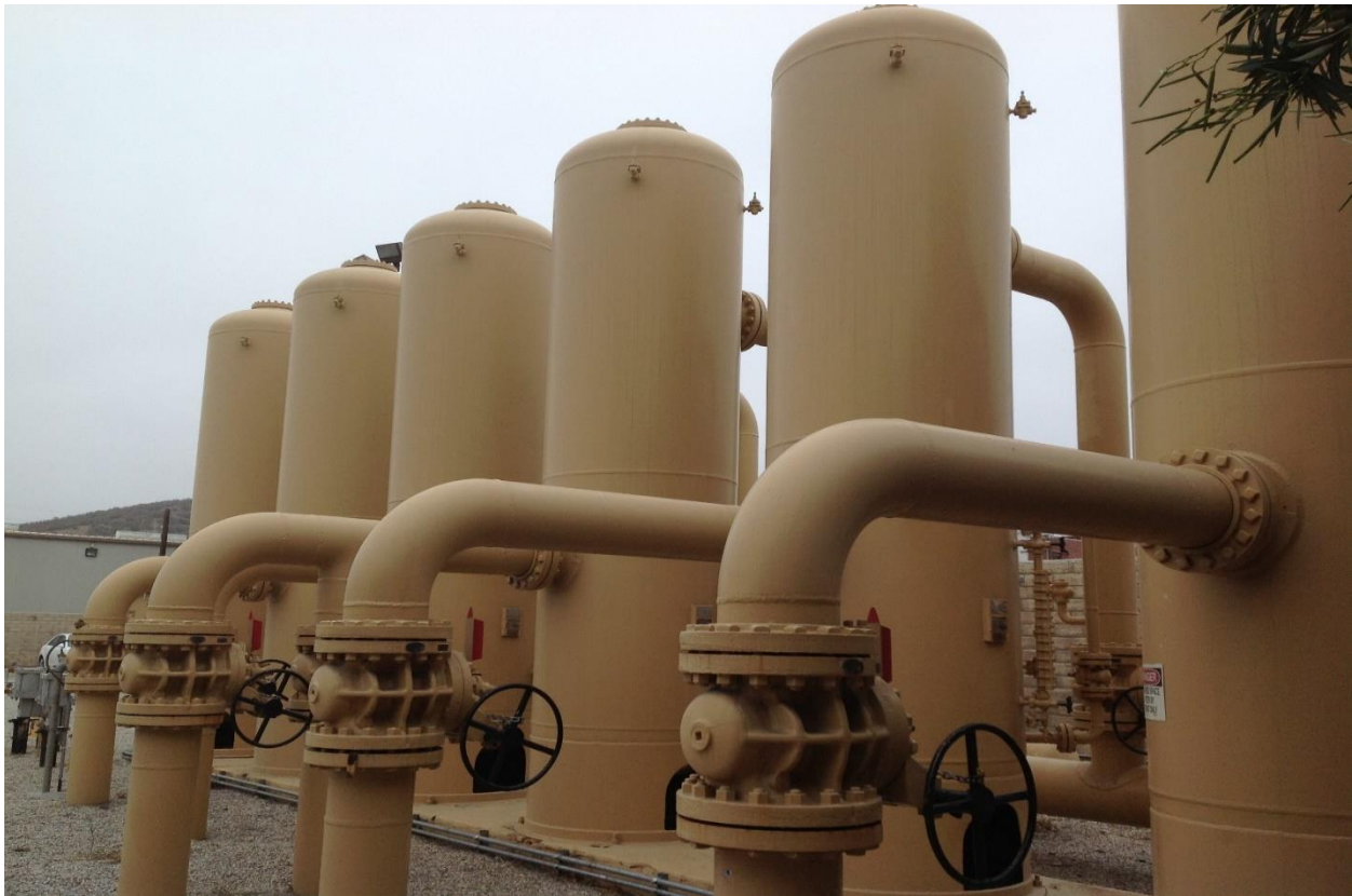
Figure 5: Existing Obsolete Equipment
