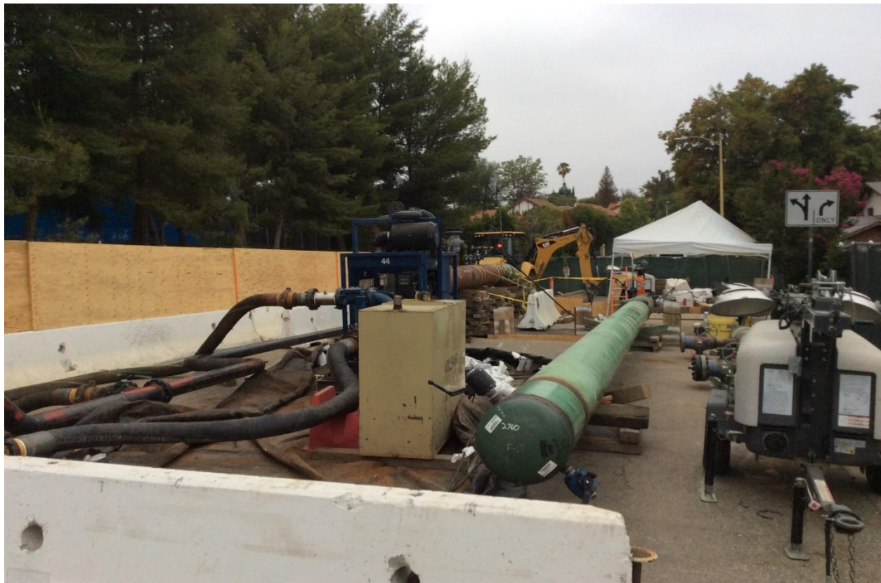
Figure 6: Pump and Test Head at Burbank Boulevard
