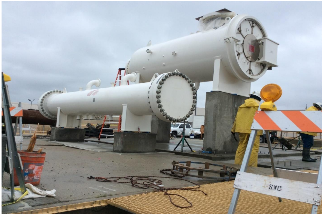
Figure 8: New Filter Separator Vessels
