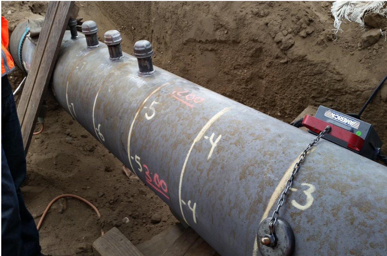
Figure 7: Fittings Installed for Gas Handling Operations at Battles Road
