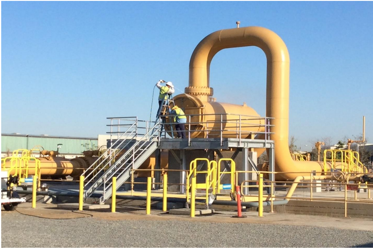
Figure 9: New Filter Separator
