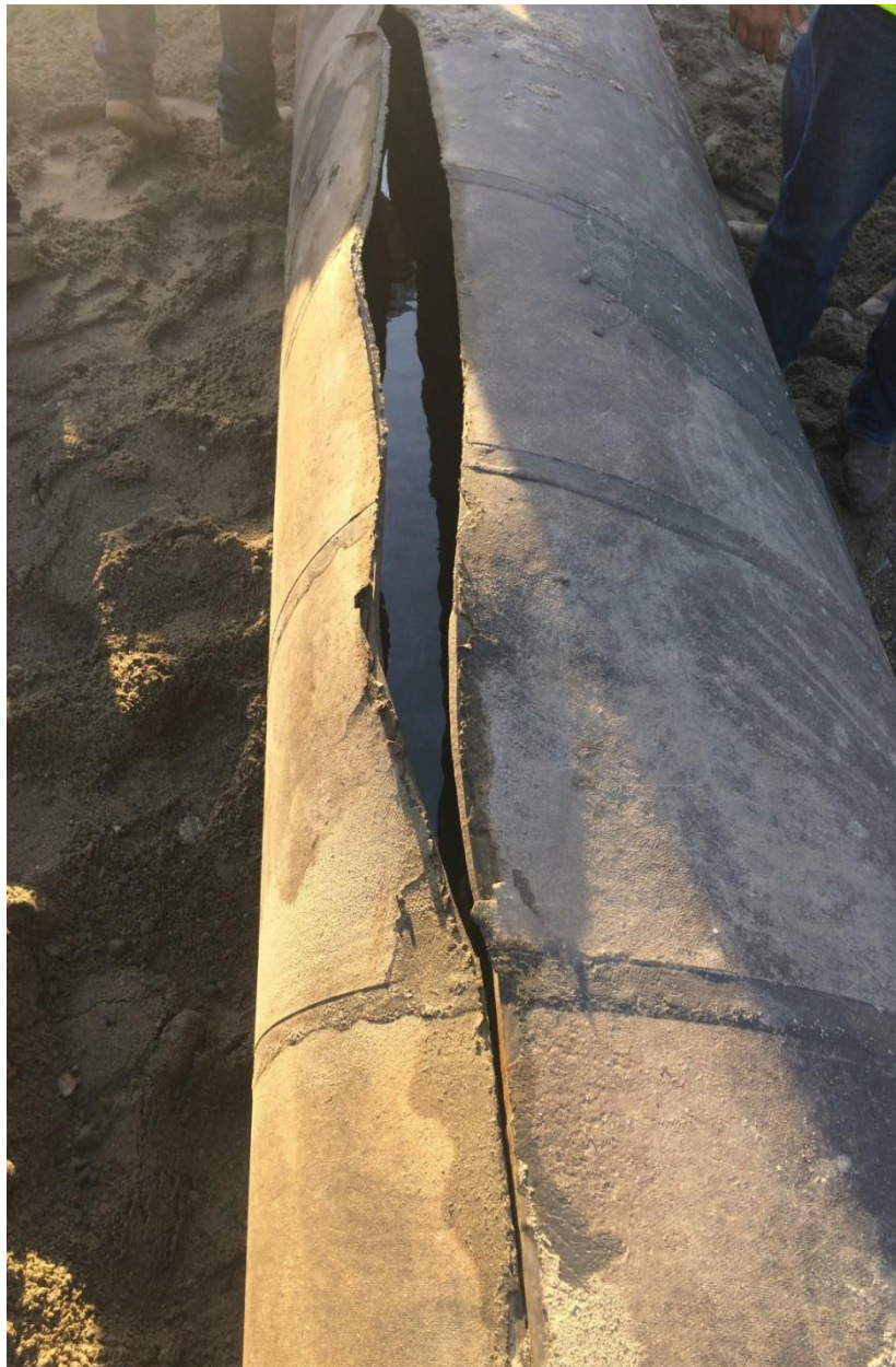
Figure 12: Hydrotest Rupture (close up)
